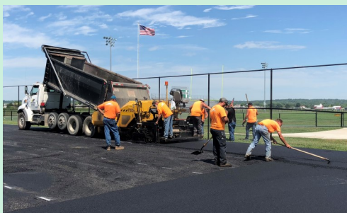
As part of our agreement with Mercy Health, the high school tennis courts are undergoing extensive renovation.
